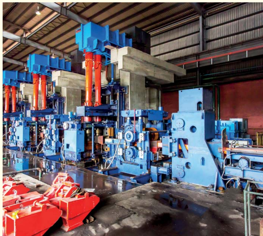
Masteel has invested in new technology to reduce its greenhouse gas emissions
