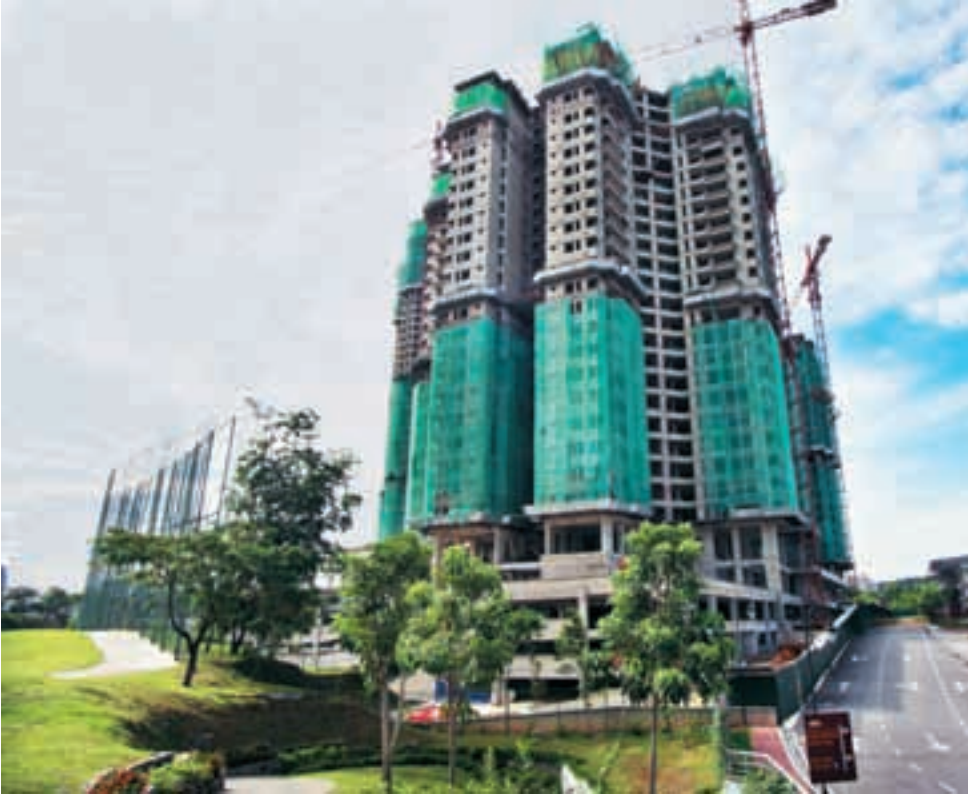
The developer had to delay the launch of its condo development currently under construction
