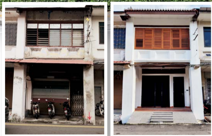
The facade of the 1920s two-storey shophouse was restored according to the Category Two heritage building requirement
